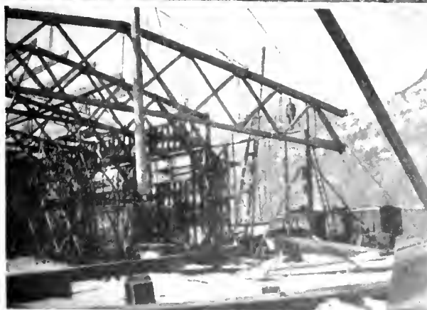
Upper—Storehouse at Great Eastern Railway terminals at Squamish, B. C. Lower—The repair shop.
